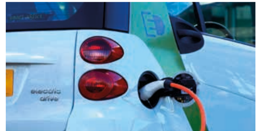
Electric car charging facilities
