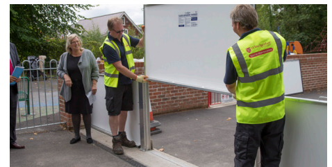
Members of the Council's special maintenance team show Cllr Horrill how the new flood gates are installed
